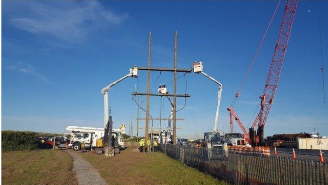
Crews work to build an overhead transmission cable as a means of repair for a massive power outage on Hatteras and Ocracoke islands. (Photo: Cape Hatteras Electric Cooperative, @CHEMC09/Twitter)
